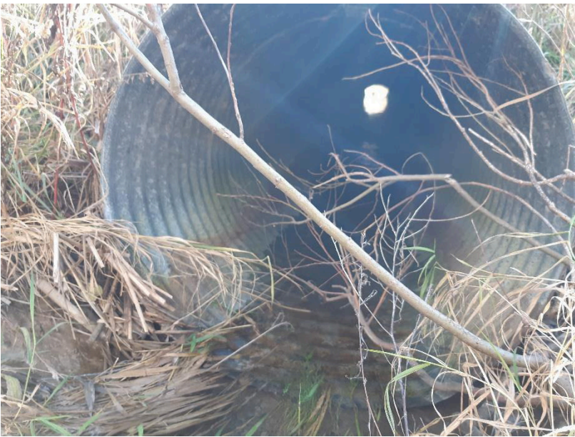
View of culvert inlet on the north side of Elgin Street East at WCC#3
