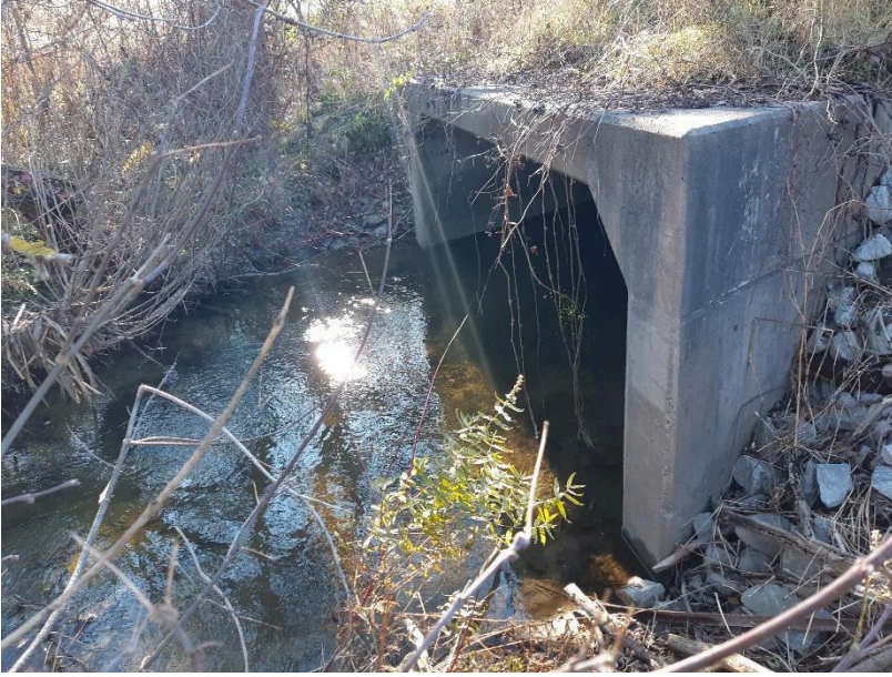
View of box culvert on east side of Brook Road North at WCC#4
