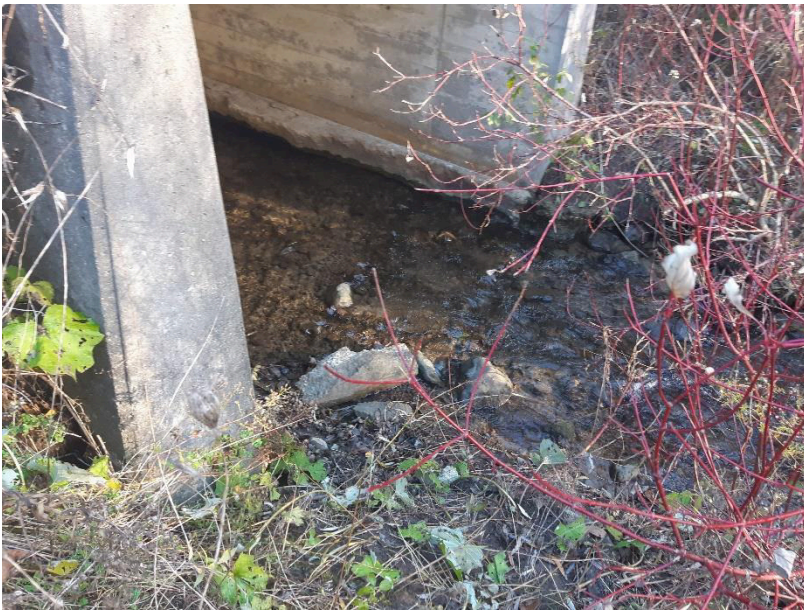
Midtown Creek – flow to south through existing concrete box culvert at WCC#1a.
