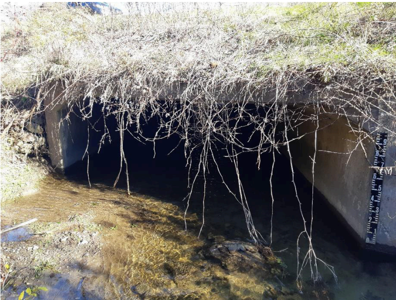
View of box culvert on west side of Brook Road North at WCC#4
